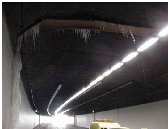
Fig 10.5.3 Bevroren lekwater over houten bekisting
