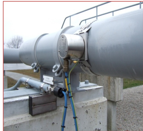
Figure 4.2 – Sand detector mounted on a flowline
