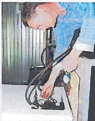
Inspection of Boilers Arco-systems
