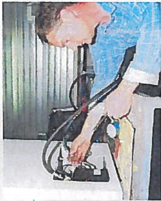
Inspection of Boilers Arco-systems
