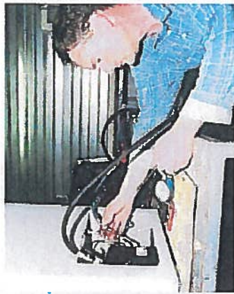
Inspection of Boilers Arco-systems
