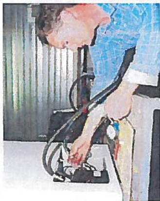
Inspection of Boilers Arco-systems
