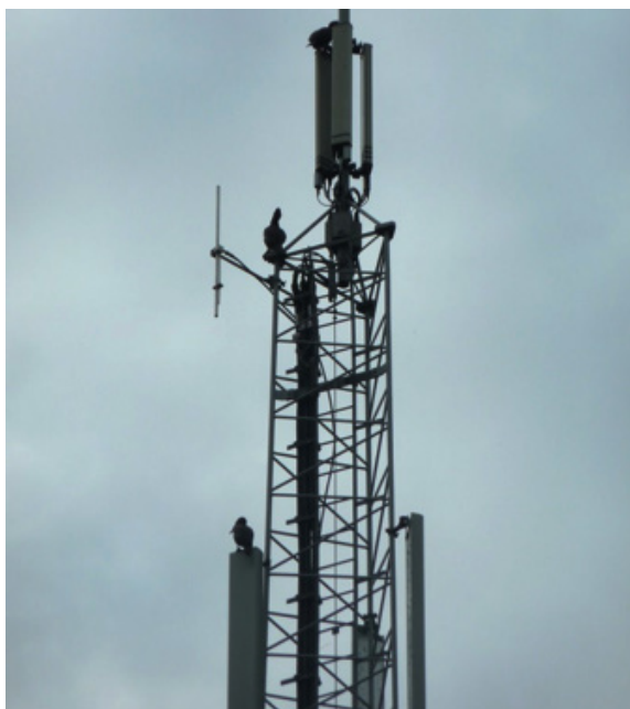
Illegale FM-antenne in mast mobiel netwerk
