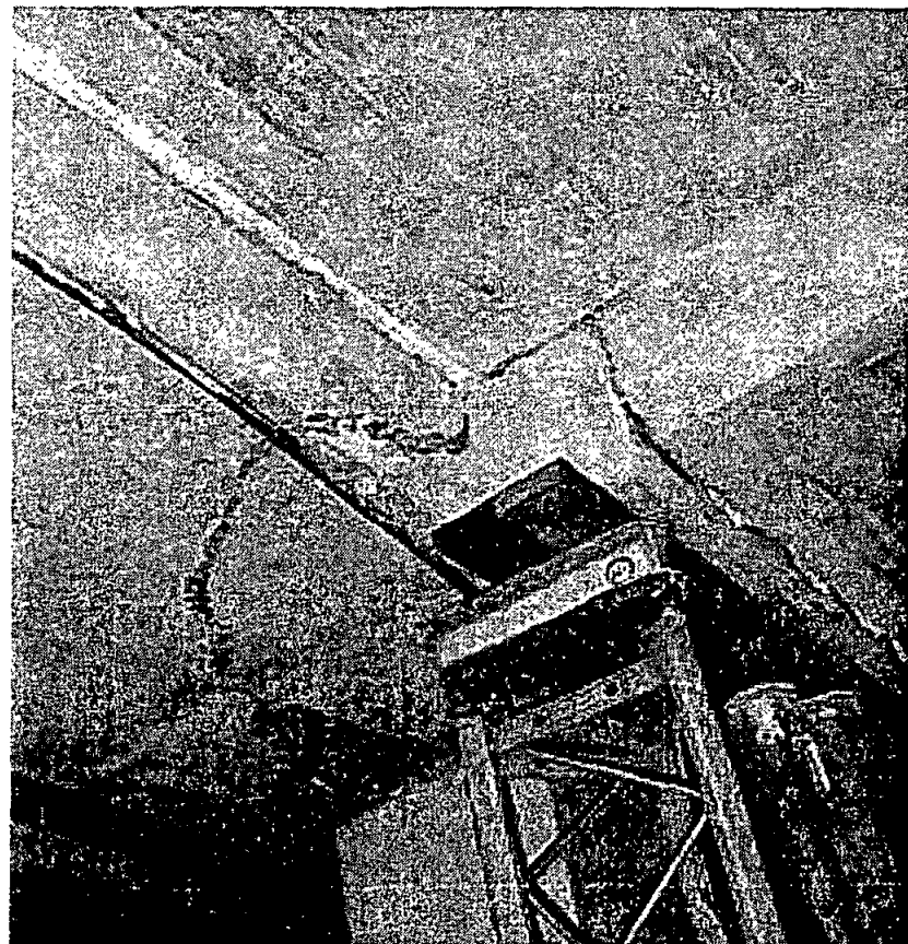
Foto 2.6: Afgebroken nok op as 11, stramien J
