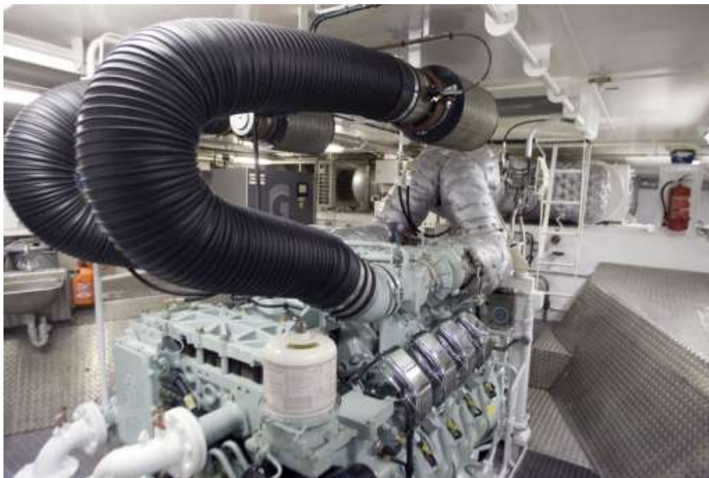
Figure 3: Retrofitting met SCR and PM filter, VT, ms Victoria.
