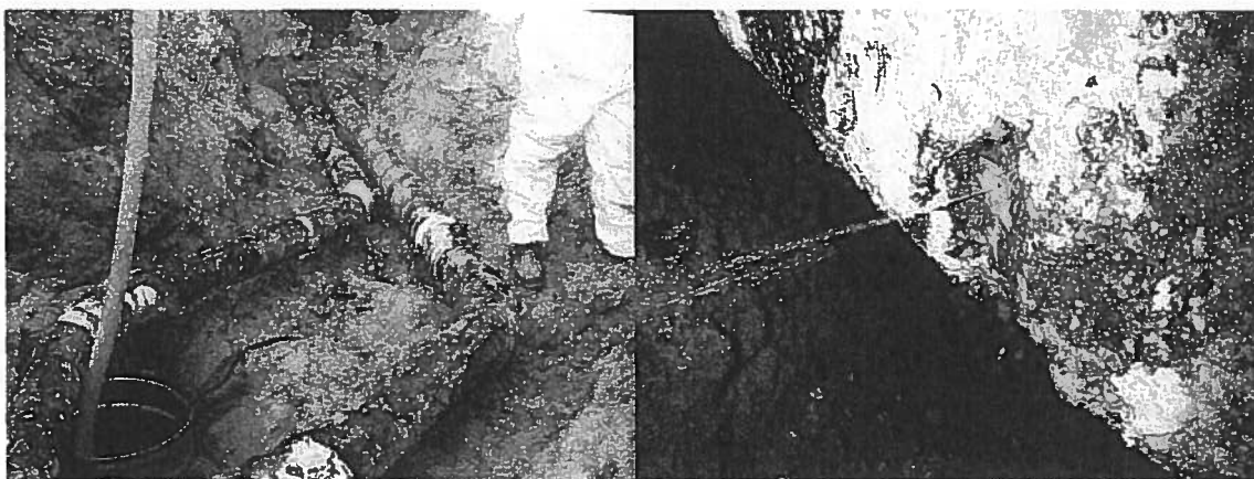
Figure 8: Uncovered basin water storage tank pipe-lines (left) and observed leak in the 4" line (right)
