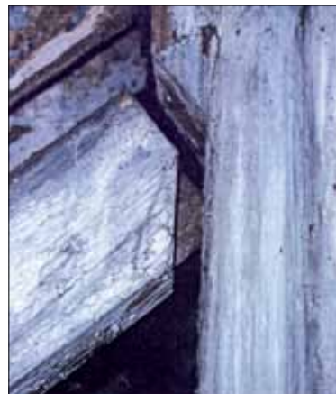
Figure A3.17 King rafter having moved and no longer adequately supported
