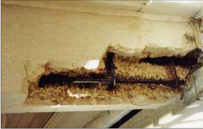
Figure A3.1 Spalling of cover/exposure of beam reinforcement
