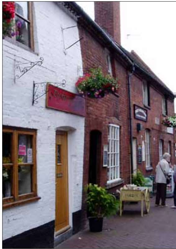
Figure A3.10 Bowing external wall, Lichfield © Brian Clancy
