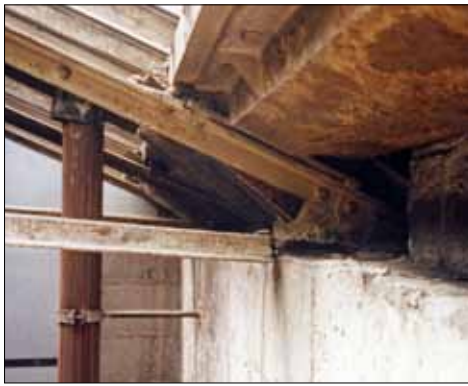
Figure A3.12 Failure of overloaded member
