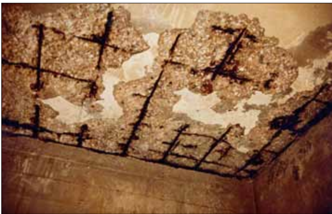
Figure A3.3 Spalling of cover/exposure of slab soffit reinforcement
