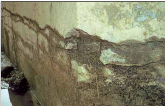
Figure A3.4 ASR in foundations
