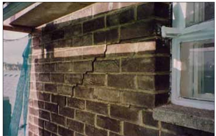
Figure A3.8 Diagonal crack following masonry joints
