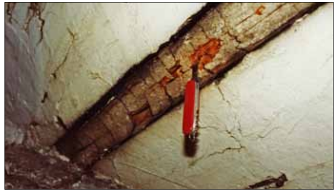
Figure A3.15 Dry rot in timber
