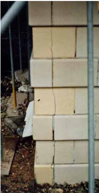
Figure A3.9 Vertical crack near corner
