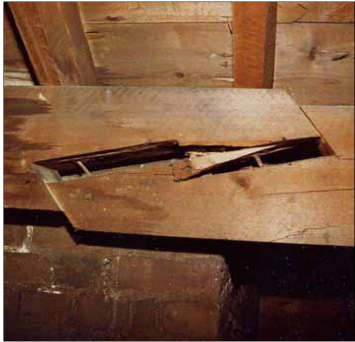
Figure A3.19 Defective joint in purlin
