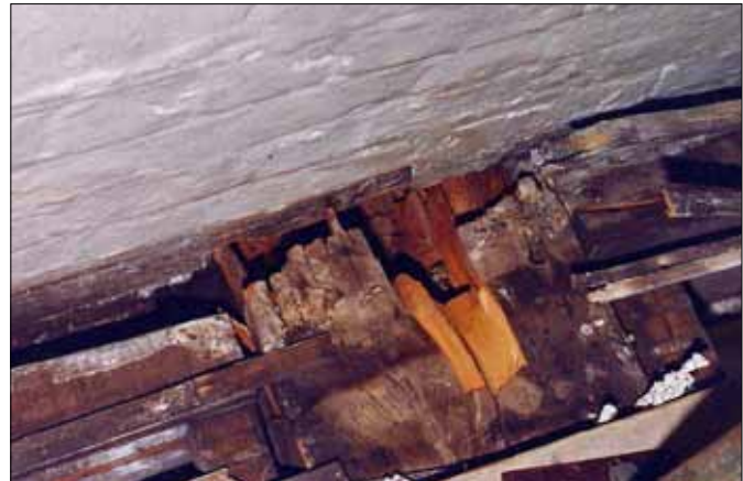
Figure A3.16 Timber deterioration
