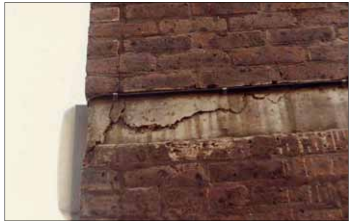
Figure A3.6 Spalling
