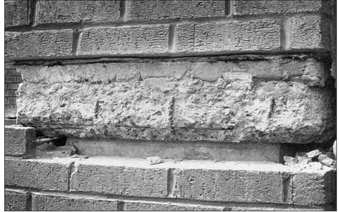
Figure A3.5 Exposed concrete in nib
