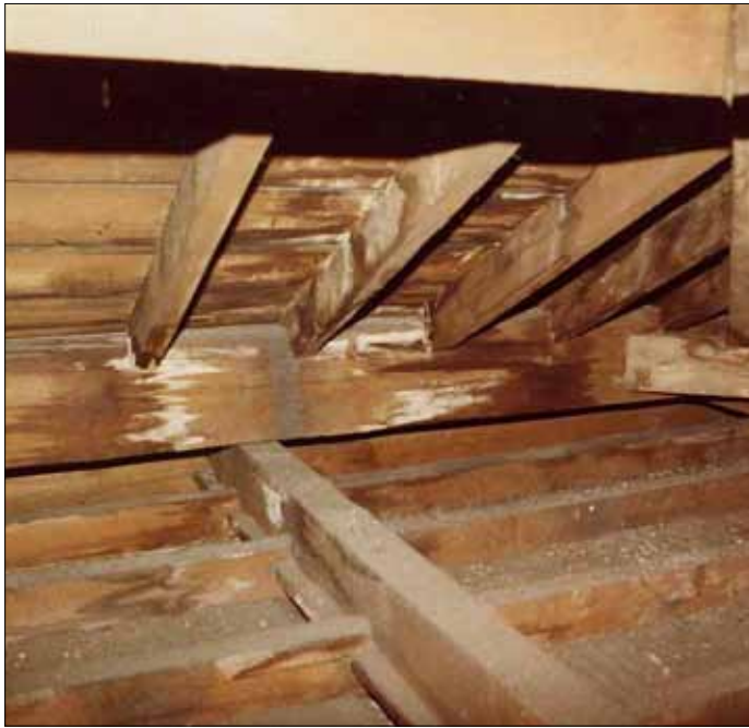
Figure A3.18 Damp staining to timbers at hip end
