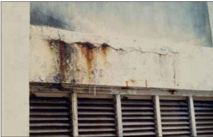
Figure A3.2 Spalling of cover/exposure of beam reinforcement
