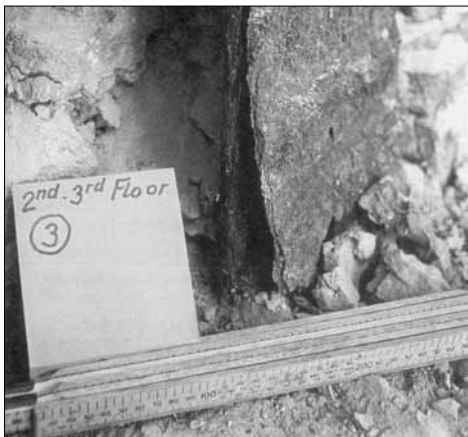
Figure A3.14 Rust flake detaching from steel stanchion
