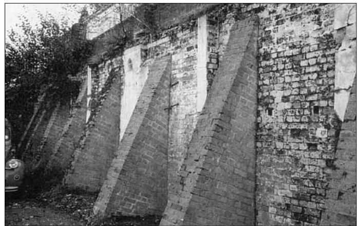
Figure A3.7 Wall out-of-plumb
