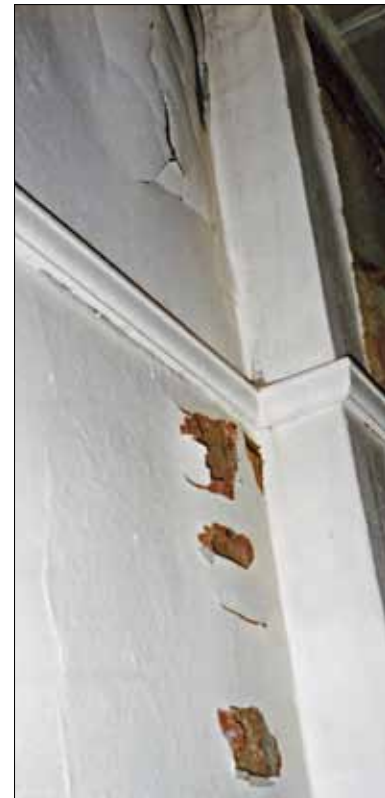
Figure A3.11 Dampness on inside face of inner leaf
